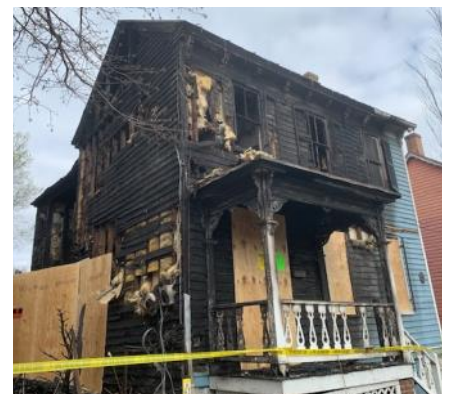
April 2020 Showing damage after fire (photo provided by Tim Youmans)
