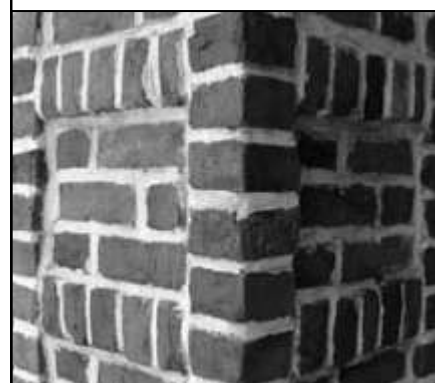
Examples of deteriorating mortar joints (top) and poor quality repointing which detracts from the wall's visual appearance (bottom).
